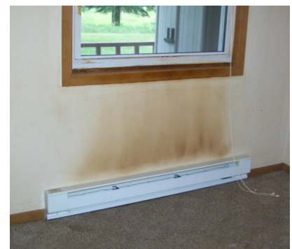
Secondhand smoke came through a wall vent and left residue behind.
